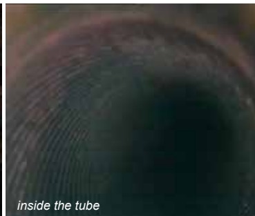
Chiller #3 Condenser Ø 67 cm, tube Ø 7/8", length: 418 cm
