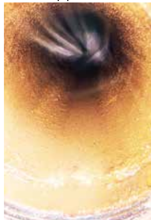
The pipe inner wall on the day when the system was installed.
