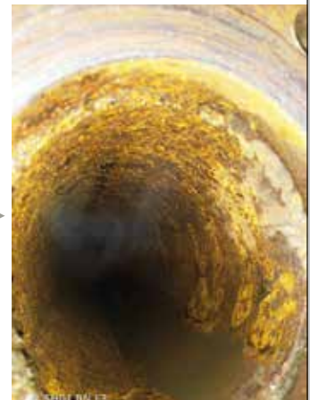
After installing the system for 3 months, the scale has been significantly reduced.
