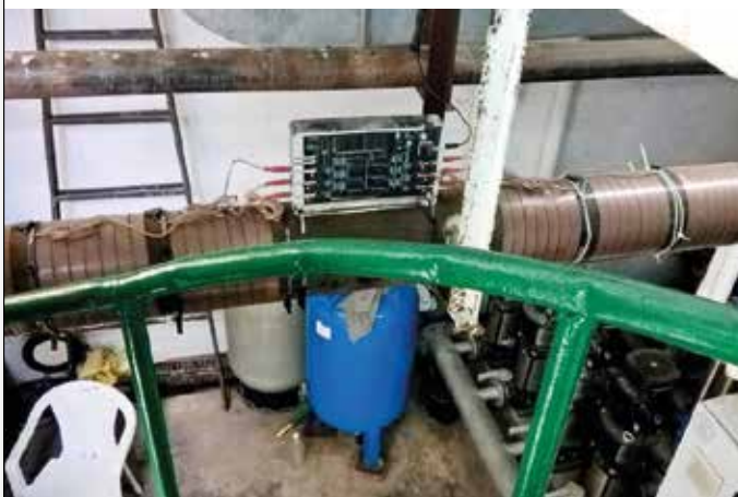
Two systems were installed.
