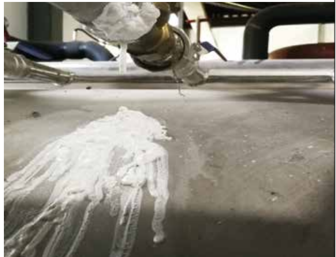
Hot spring water flows out of the pipe joint, it builds up stalactite-like scales over time.
