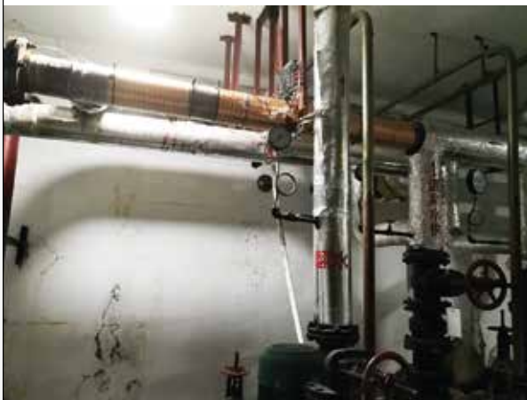
The hot spring water pipeline is far away from the villa, so the water has to be pumped. The unit was installed on the delivery pipe.
