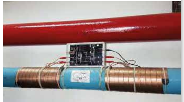
Anti-Scale System installed
