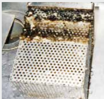
The status after being used without cleaning since the installation in June (no adhered materials are seen on the portions usually contacting with water).
