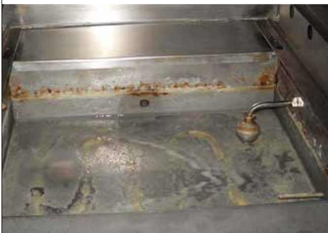
Pan before the installation, hard calcium and etched line present.
