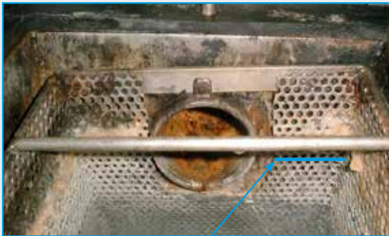
Usual level of standing water.
