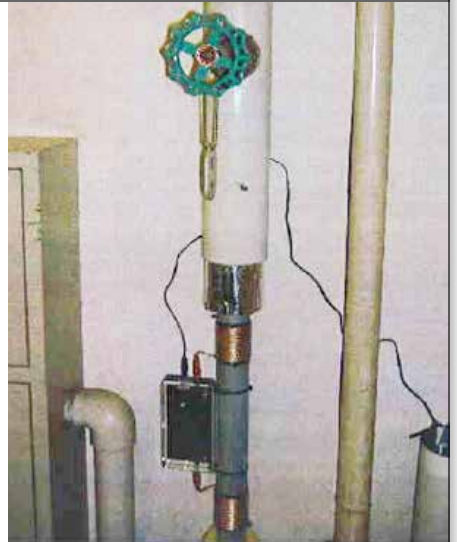
The unit was installed in the factory kitchen
